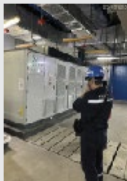
Supply of medium-voltage Drives for Vung Ang Thermal Power Plant
