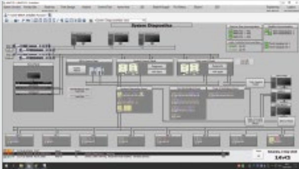
Supply of DCS for Fuel hydrant system at Terminal 2 area of Noi Baif International airport
